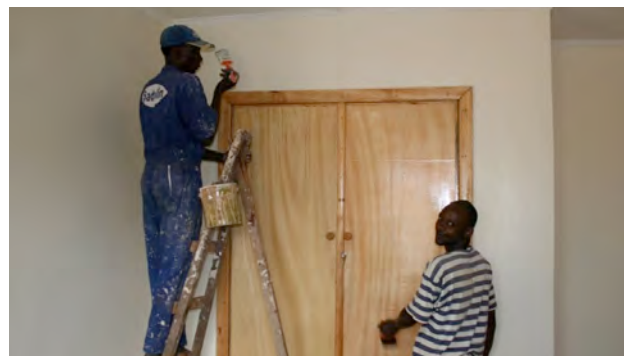
WALLS, CEILINGS, AND CUPBOARDS GETTING THEIR LAST COATS OF PAINT AND VARNISH
