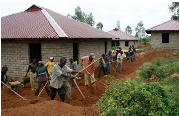
EXCAVATION BEING DONE AROUND THE COTTAGES IN ORDER TO CONTROL THE RAIN WATER RUNOFF
